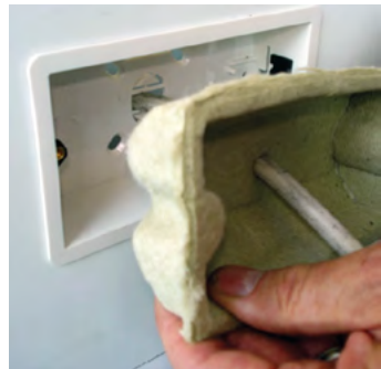
Intumescent pad being installed in a dry lining box (Photo courtesy of Knauf Drywall).
