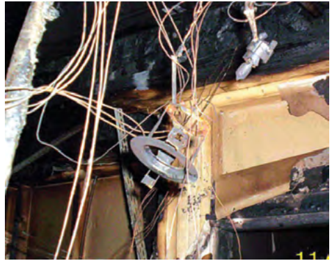
Result of a downlighter fire (Courtesy of Manchester City Council - Building Control).
