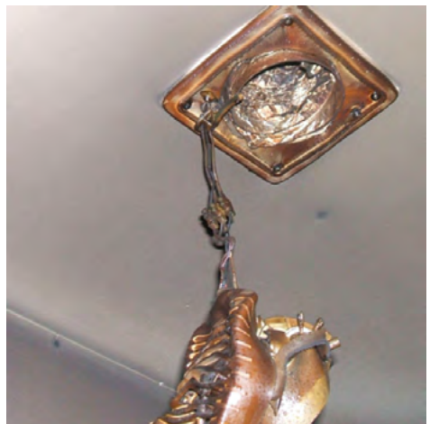
Fire spread into bathroom via plastic duct (Photo courtesy of Greater Manchester Fire & Rescue Service).
