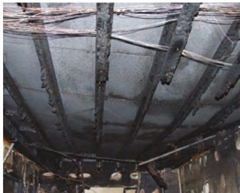
Result of an eight minute fire on lightweight joists (Courtesy of Manchester City Council - Building Control).
