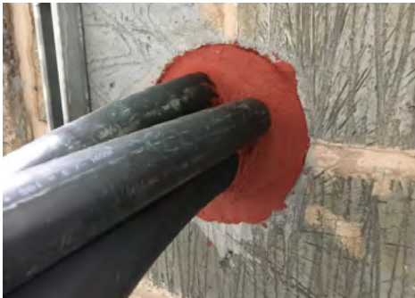
Fire seals around cables and trunking.
